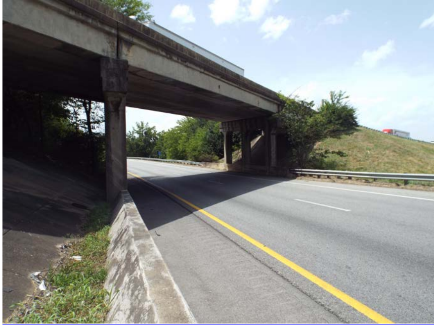
CLEARANCE - AHEAD I75 UNDERPASS
